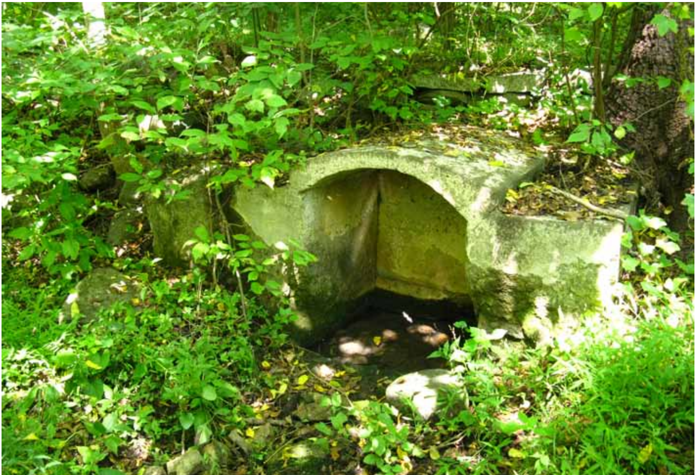
Part of the old spring box remains on the former Bolen land.
